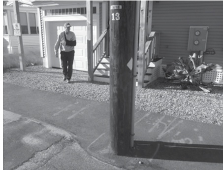
Figure 4-32: Make sure all utility lines are clearly mark during the project layout phase.
