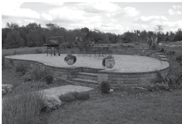
Figure 4-4: Excessive slope on a patio will create a noticeable lean on chairs and tables.
