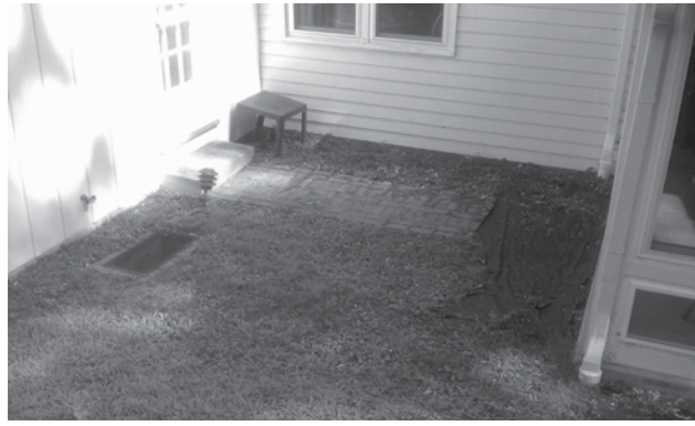
Figure 4-6: Take pictures of the exterior and interior of the foundation walls to document their condition before you move equipment or materials on site.
