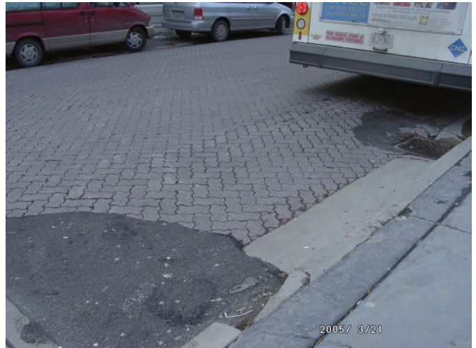
Figure 26. Patching compromises the structural integrity of ICP and occurs when proper maintenance techniques are not followed.
