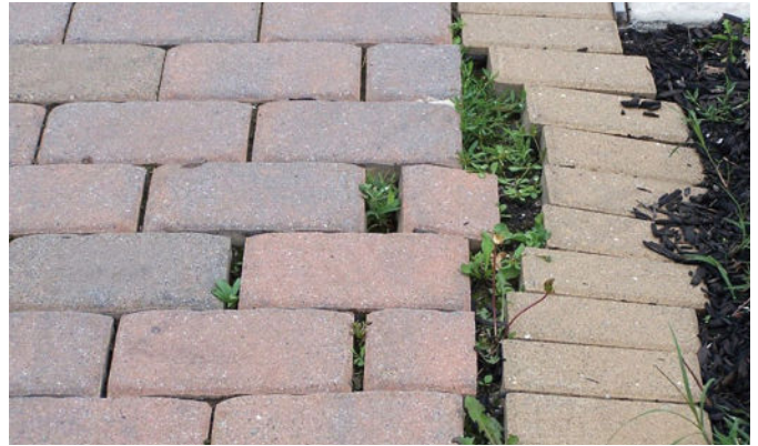
Figure 19. Lack of an effective edge restraint has allowed the pavers to separate and compromise the structural capacity of the ICP.
