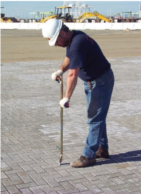
Figure 41. An alignment bar and string line can be useful to tweak the pattern and make it line up with the surrounding undisturbed paver.
