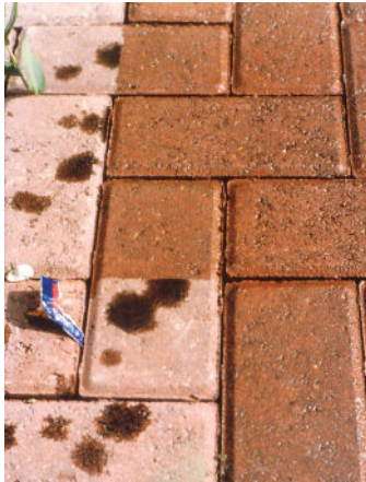
Figure 3. It is easier to remove oils stains from pavers that have been sealed.
