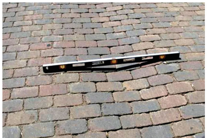
Figure 27. Rutting occurs when the underlying layers settle. The extent of rutting is easily measured by laying a straight edge across the rut.
