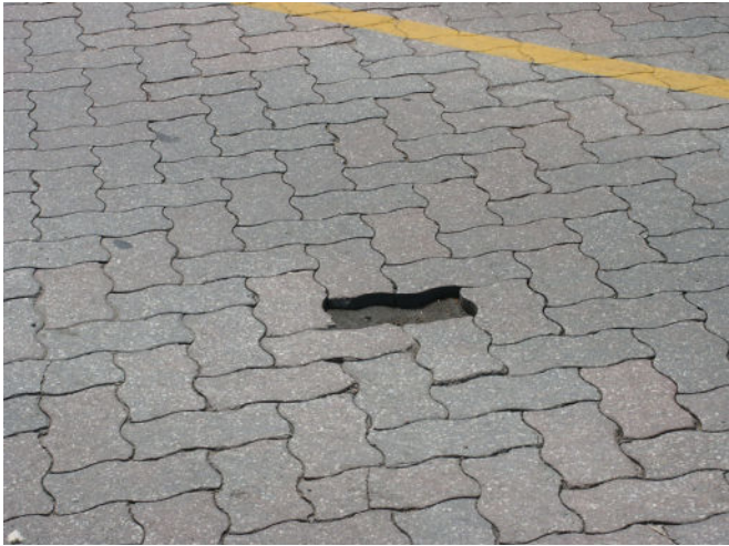
Figure 25. Missing pavers should be replaced as soon as possible to avoid damage to the surrounding units.
