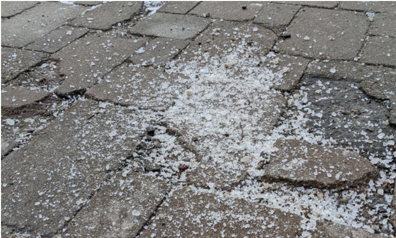
Figure 8. Use deicing chemicals sparingly and remove any excess after it has completed its job.
