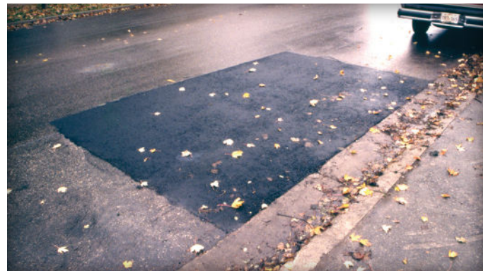
Figure 7. Pavement damage from settlement and shrinkage of cold patch asphalt.
