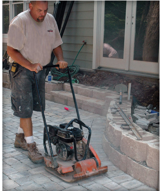
Figure 9. Final compaction of the pavers and settling of the sand into the joints.
