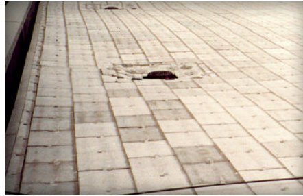
Figure 4. Some ballast-type slabs for roof decks are made with lightweight concrete materials. They can be joined with tongue-and-grooves and/or with connectors to resist wind uplift. This is one of several designs available.
