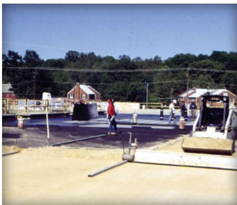
Figure 19. A mechanical screed used to level bedding sand on a roof parking deck project.
