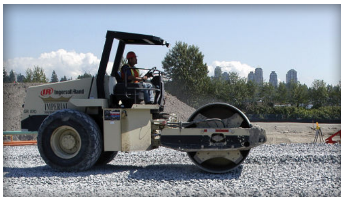
Figure 15. A 10 ton (9 T) vibratory roller compactor settles ASTM No. 2 stone subbase for a large shopping center parking lot.
