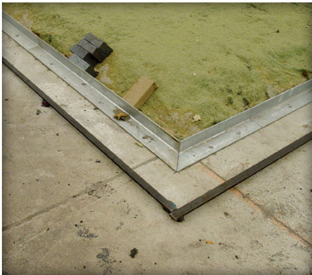
Figure 17. On larger projects, thick steel screed bars are placed on the concrete base to ensure a uniform bitumen-sand bedding thickness.
